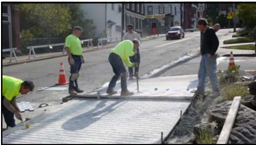
Rick DeCarlo and crew stamped a brick pattern for the new sidewalks alongside Mały Park.
